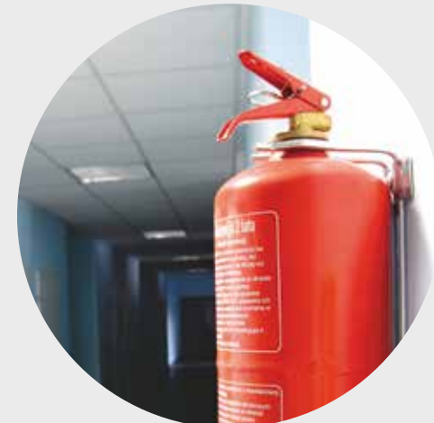
Fire Fighting System
